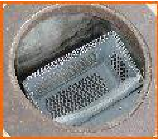
Curb Inlet Basket (CIB)
