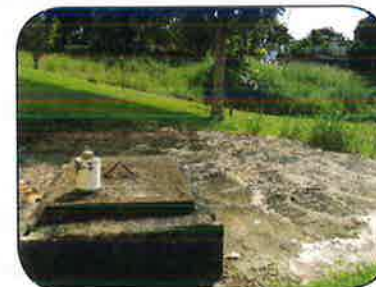
Keep septic tanks sealed.
