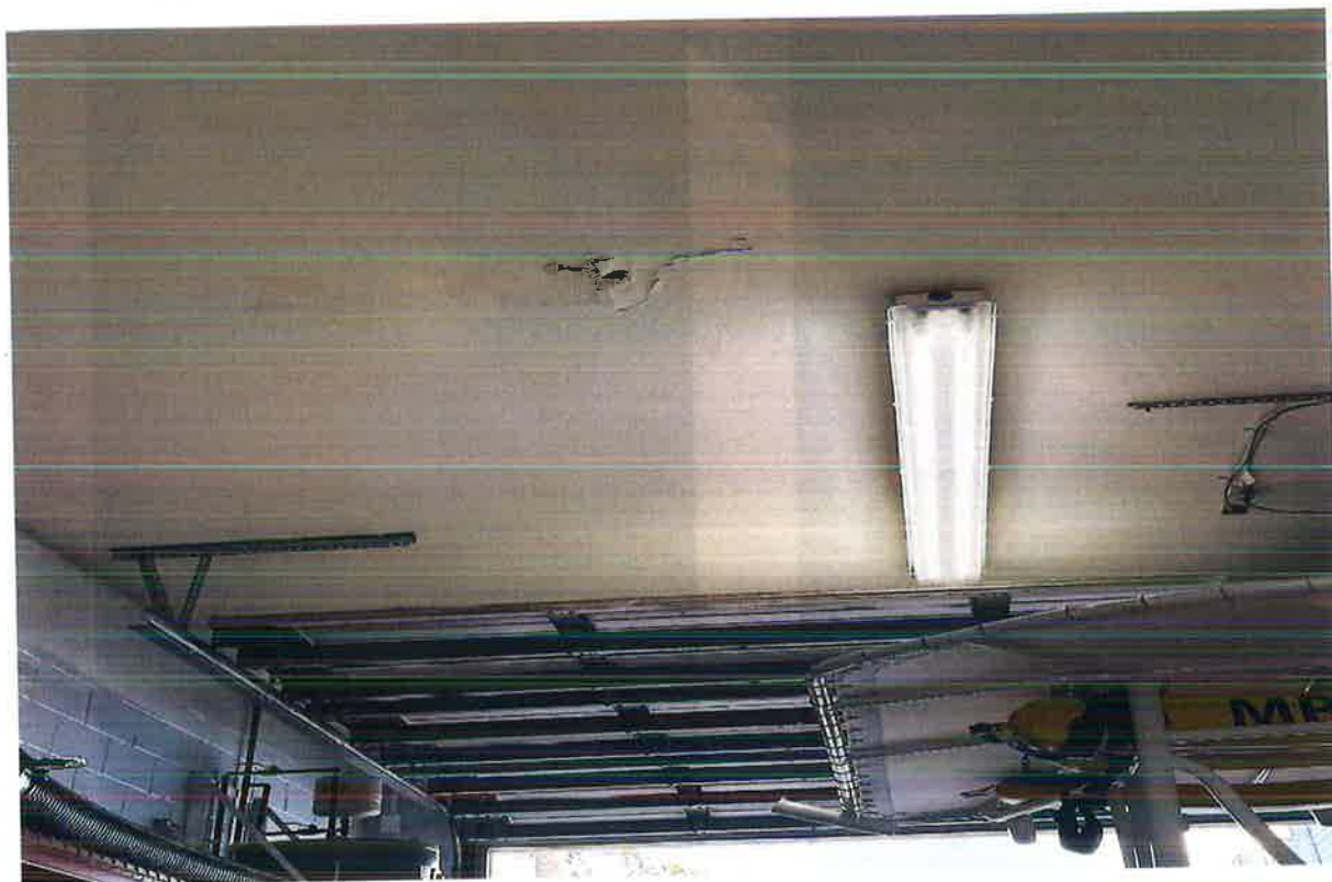
Attachment 2: Leakage in fire engine bay
