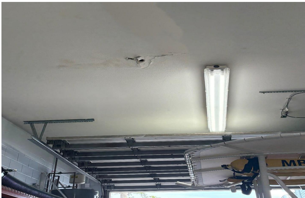
Attachment 2: Leakage in fire engine bay
